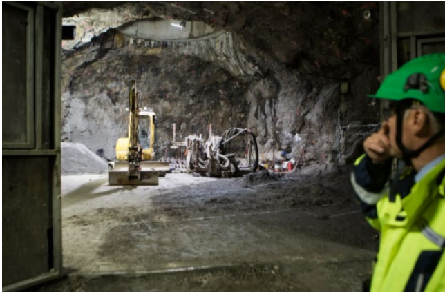
Excavating equipment at the site of the Onkalo repository project, the world's first permanent spent-nuclear-fuel storage facility, deep in granite bedrock in Finland, in 2017.
